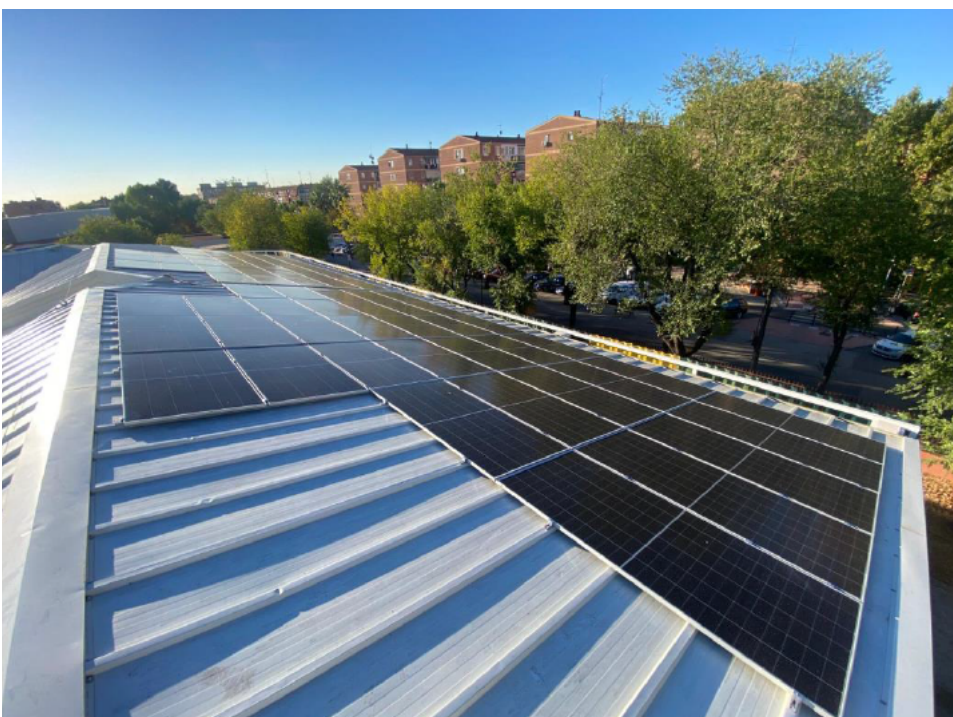
The energy community's first municipal installation on the Civic Centre Las Margaritas (40 kWp) © Getafe
